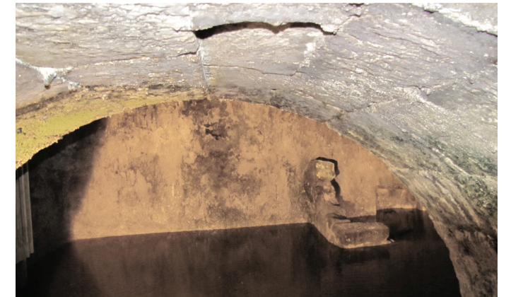
The arch and vaulted ceiling built by Hadrian over the Hasmonean water reservoirs. The Romans built a market square at ground level above these arches over the pool.
